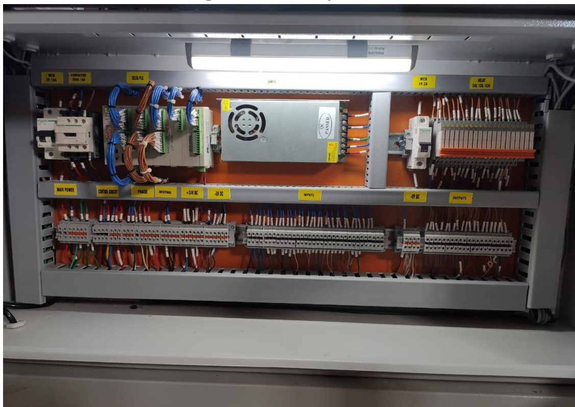
Fig 3.3.1 Panel board wiring
